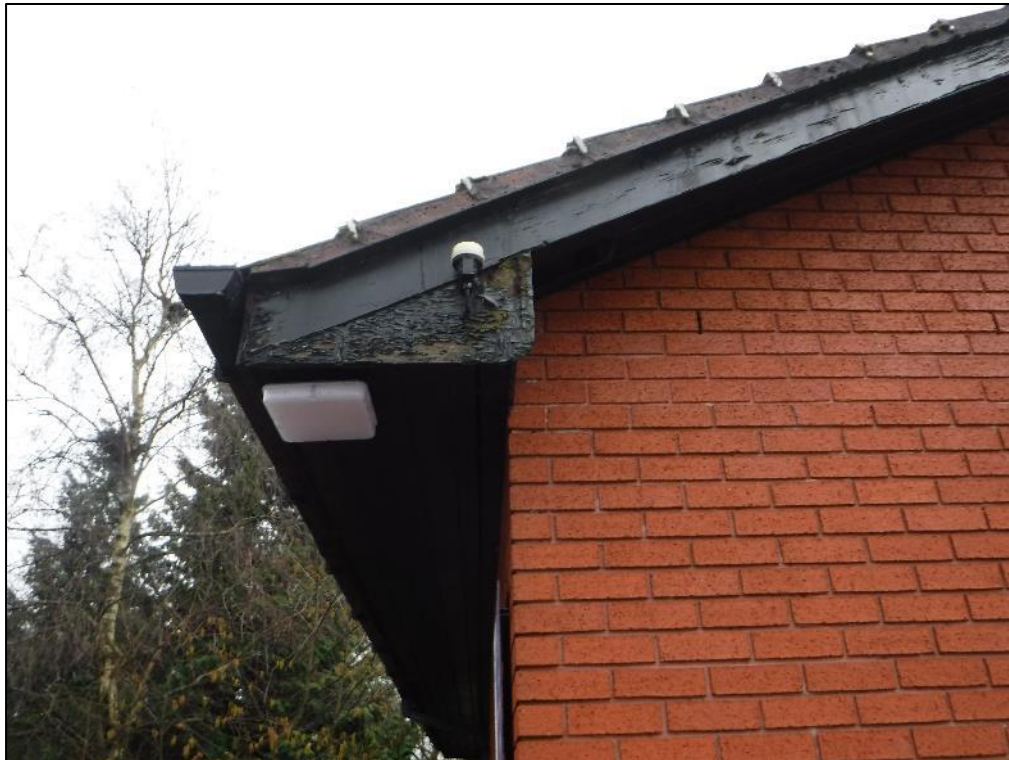
Photo 18 – Soffit at east gable of Building B15.
